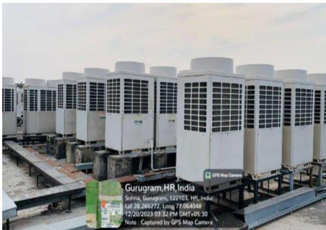
VRV Systems (Outdoor Units)
